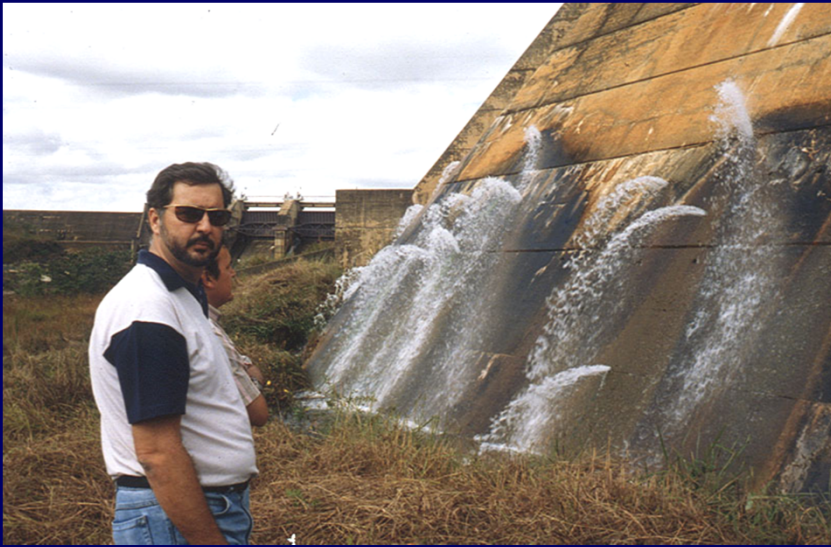
(Concrete Dam Leaking!)
