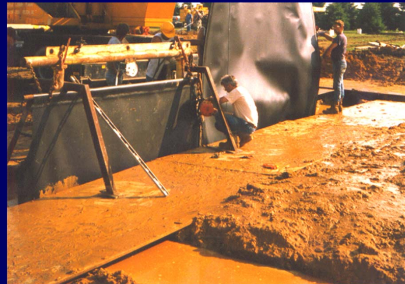
(Placement of GM Panels)
