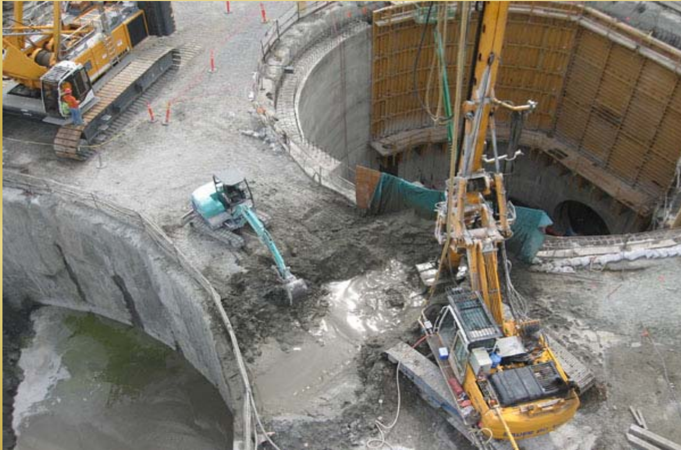
Jet grouting stabilization at TBM break-out locations for construction of a new sewer tunnel at the Brightwater Treatment Plant in King County, WA.
