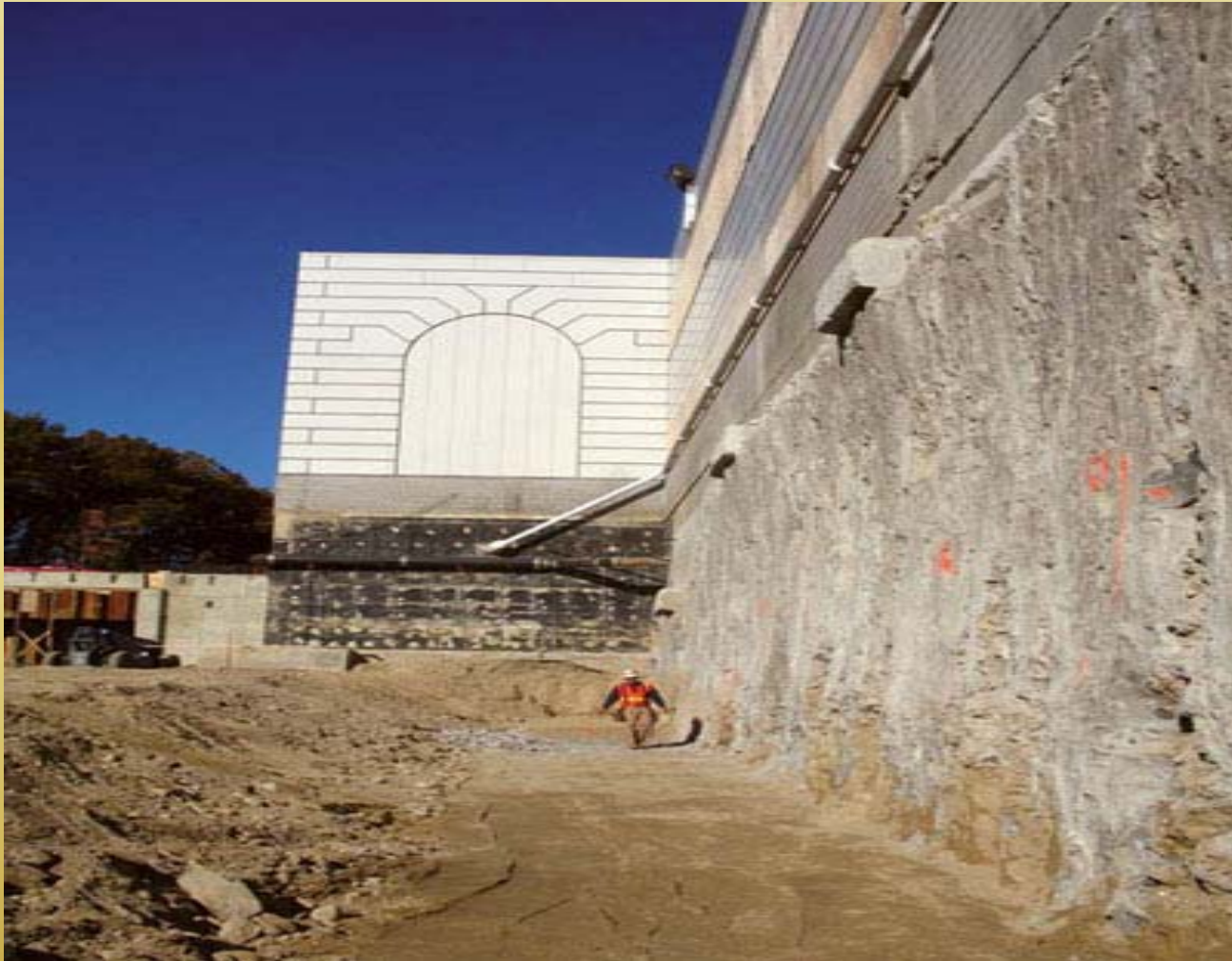
Jet grouted soilcrete columns to underpin and provide excavation support for this wall at the Bayer Healthcare facility in Walpole, MA.
